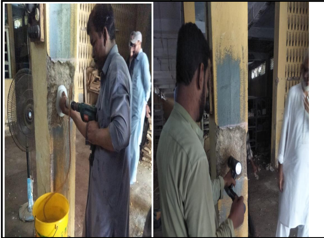
Figure-01: Drilling for cutting 0.5" dia concrete core prior to Capo Test at Location
